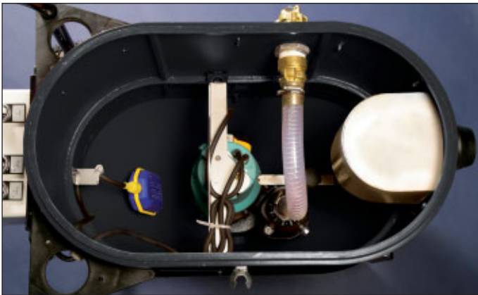
Inside view with installed pump and float switch for suction engine and pump.
